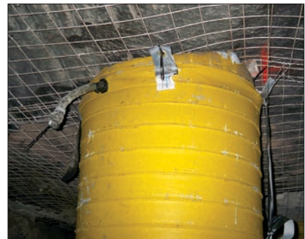
Pumped full and pressurized.
